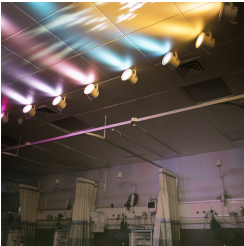
Computer Controlled Lighting Installation (2009)
